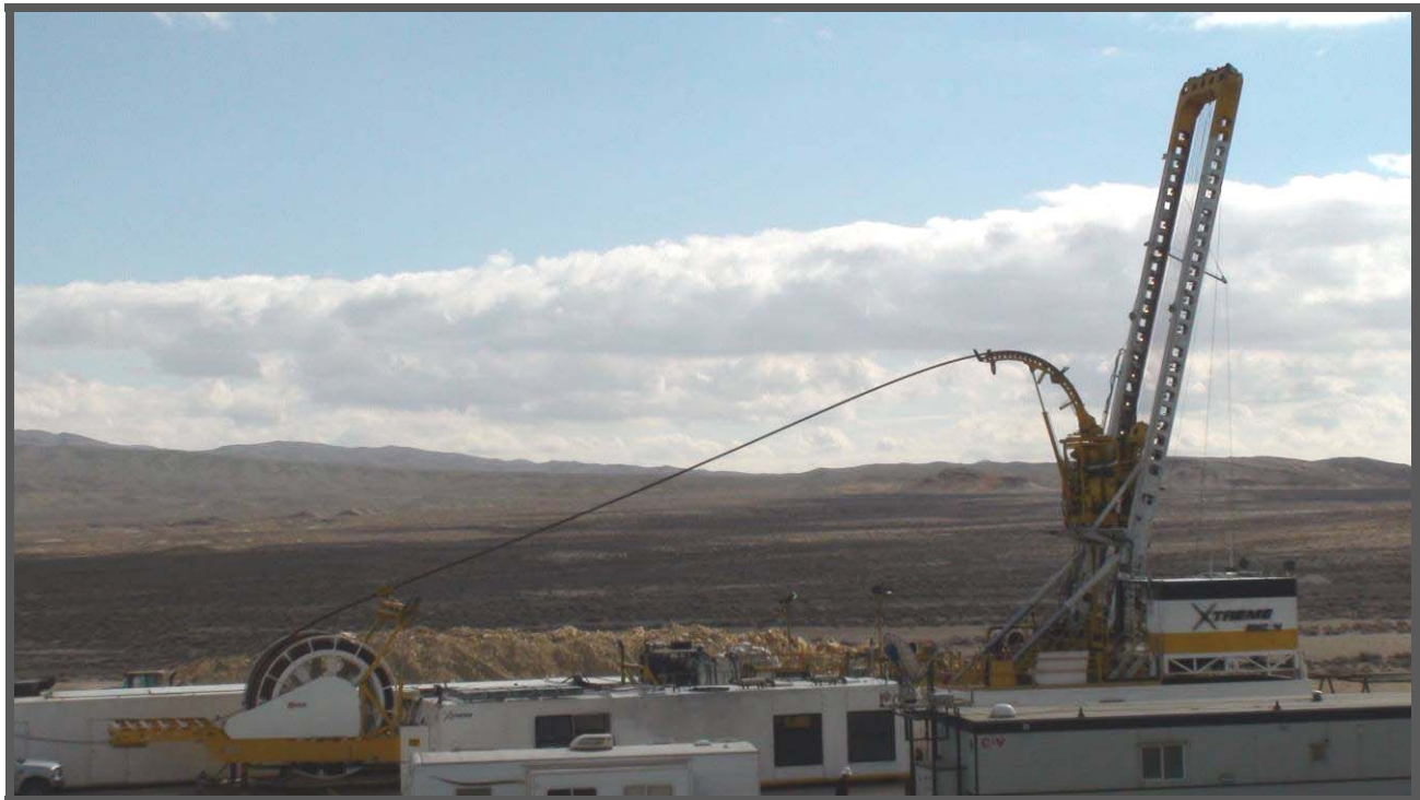
Xtreme Coil Rig #4, an XTC 200DT, drilling a deep geothermal well in Nevada
